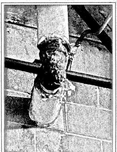
Shown above is an example of the old, rusty piping inside the walls of the existing RCMS building.
