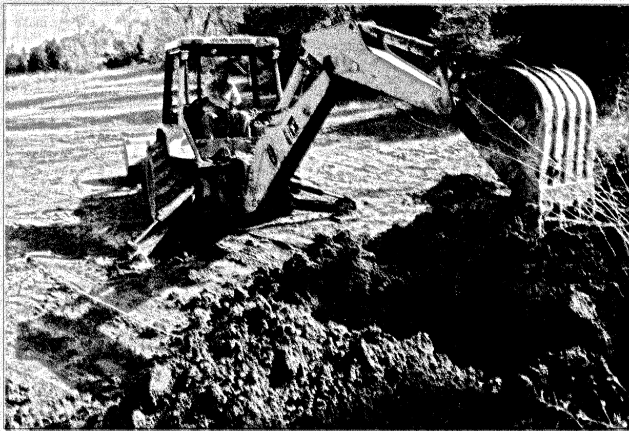
Mt. Vernon city employee Jordan Bales was busy Tuesday removing dirt at Lake Linville Park in Mount Vernon as part of many planned projects for the area. According to city officials, a new concrete basketball court is coming soon and a new volleyball area is already complete. There is also talk by council members of constructing rental cabins as well as shelters and walking paths. All of the projects are expected to take several years to complete but many are underway now. (See related story on page B1 for more details)
