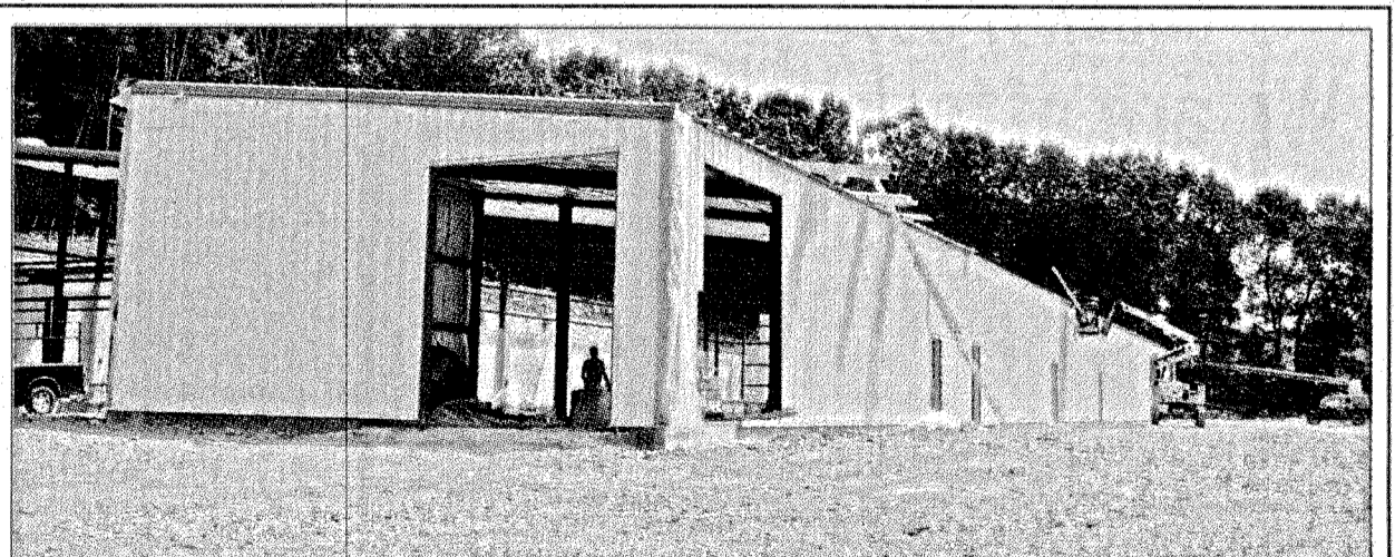
The siding and the roof are being placed on the new Microfoodery Plant on Richmond Street making the building visible from the road. According to officials, construction is on schedule and the plant plans to soon have a website where job seekers may apply for a position. The website address will be announced once owners are ready to begin hiring.
