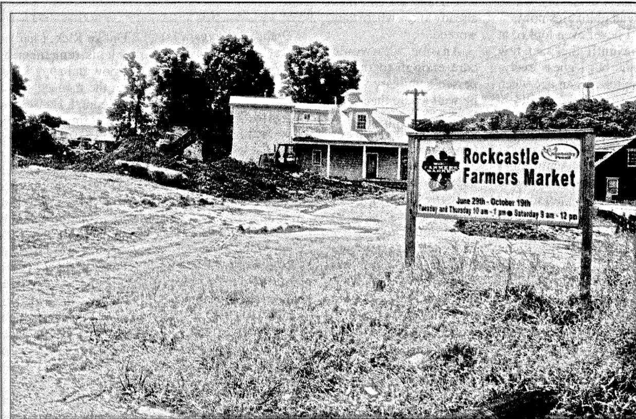
Goff Excavating was busy this week working at the site of the proposed Farmers Market on Richmond Street in Mount Vernon. Officials say bids for the project were surprisingly high and the building size may have to shrink to bring the project in under budget.
