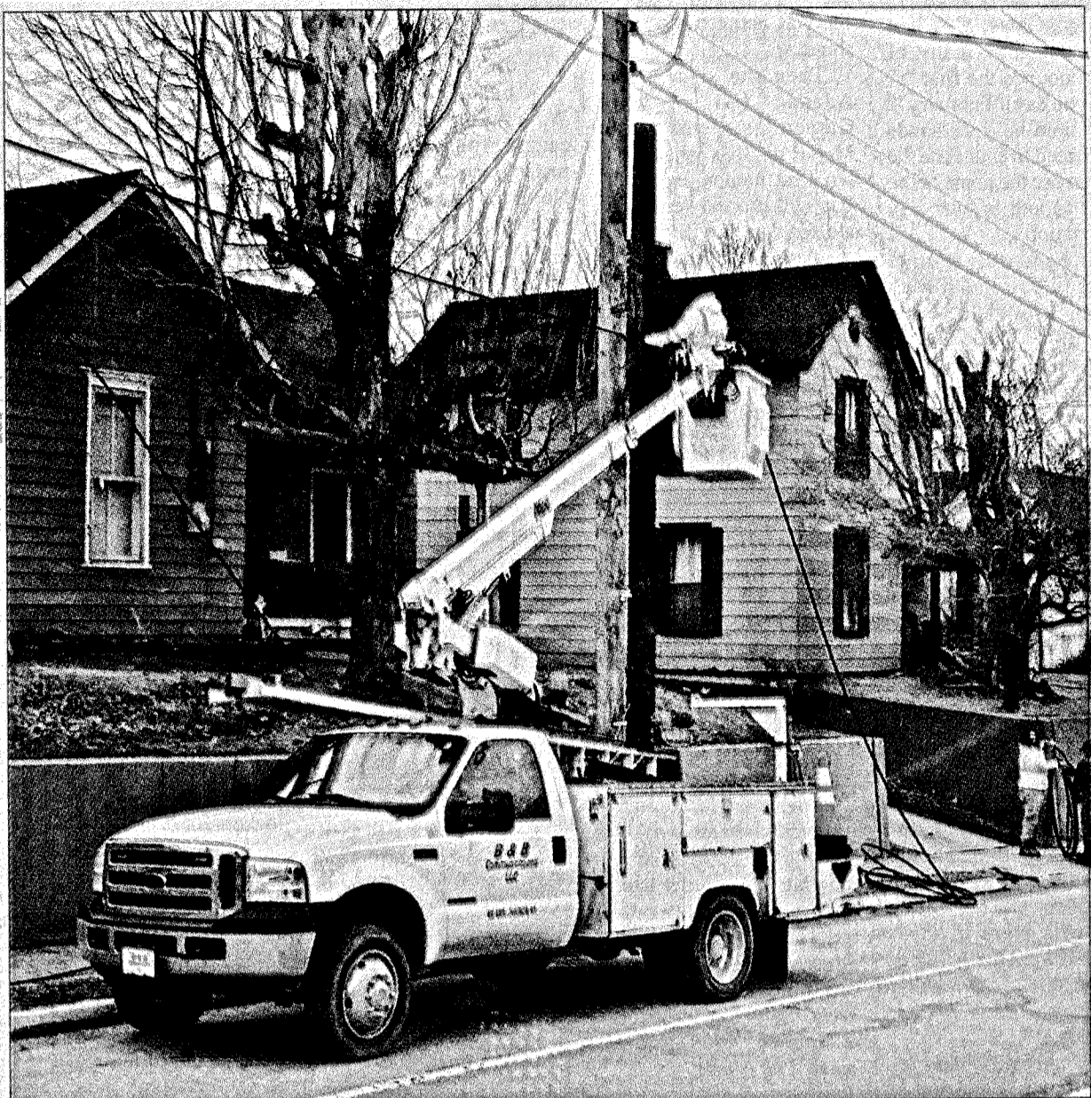
B&B Communications, out of Hazard, is busy installing TV cable in Livingston. According to Livingston Mayor Jason Medley, the company, which is already hooking up customers in Livingston, will eventually reach 200-300 customers in Livingston and surrounding areas.
