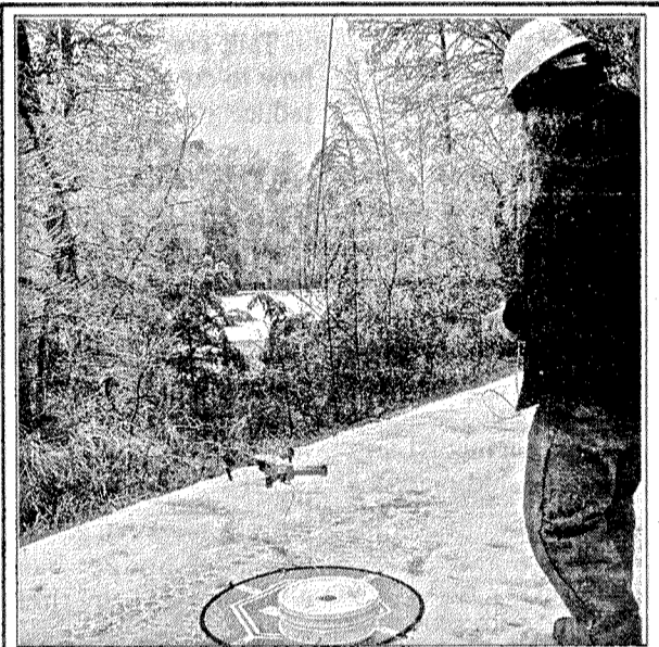
Jackson Energy Drone Pilot/Staking Supervisor Seth Jones prepares a drone to pull a rope across the pond on Madison View Lane in Rockcastle County so crews can pull the new wire necessary to restore service. Photo courtesy of 1st Class Line Tech Brent Johnson.
