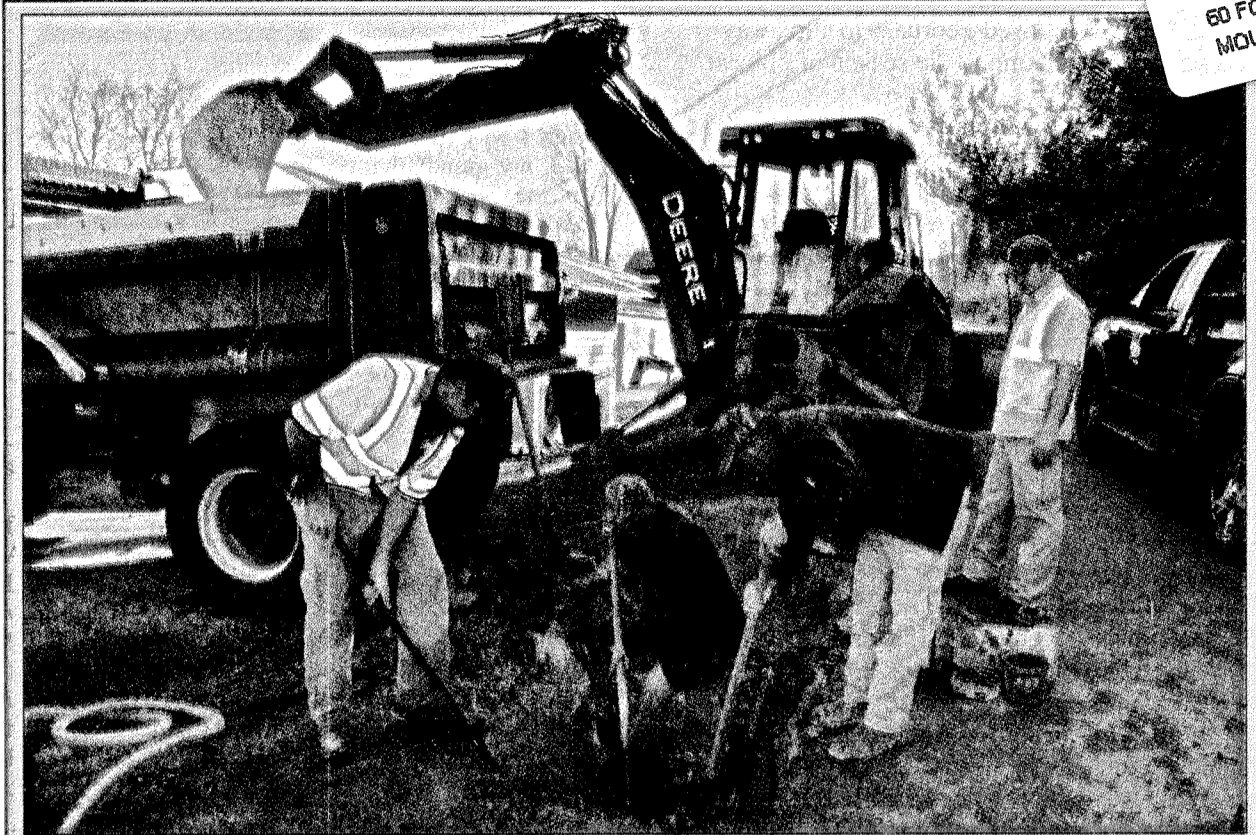
Mt. Vernon City employees jackhammered concrete and dug out a water leak on Richmond Street Tuesday morning. Frank Baker, Maintenance Department Supervisor, said the leak was caused by an older fitting breaking loose and crews were able to repair the leak quickly. According to Baker, only McDonald's was affected by the leak but the restaurant was back in business a few hours after the leak was discovered. Several water lines in Mount Vernon are older and may have fittings that could break loose anytime but Baker and his team are keeping a close eye on areas where lines are older. Baker said this leak had nothing to do with recent temperature changes.
