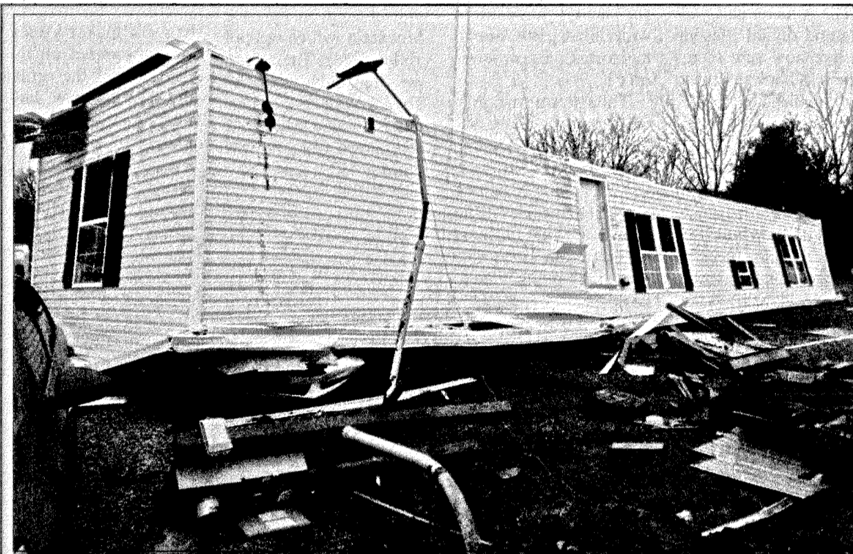
This mobile home was torn from its foundation and flipped over onto its top during Saturday's heavy storms in the Brindle Ridge area. Officials say the home rolled onto a car in the driveway and two occupants were inside the home when it rolled. However, neither occupant was injured. Reports of wind damage came from all areas of the county but no injuries were reported.
