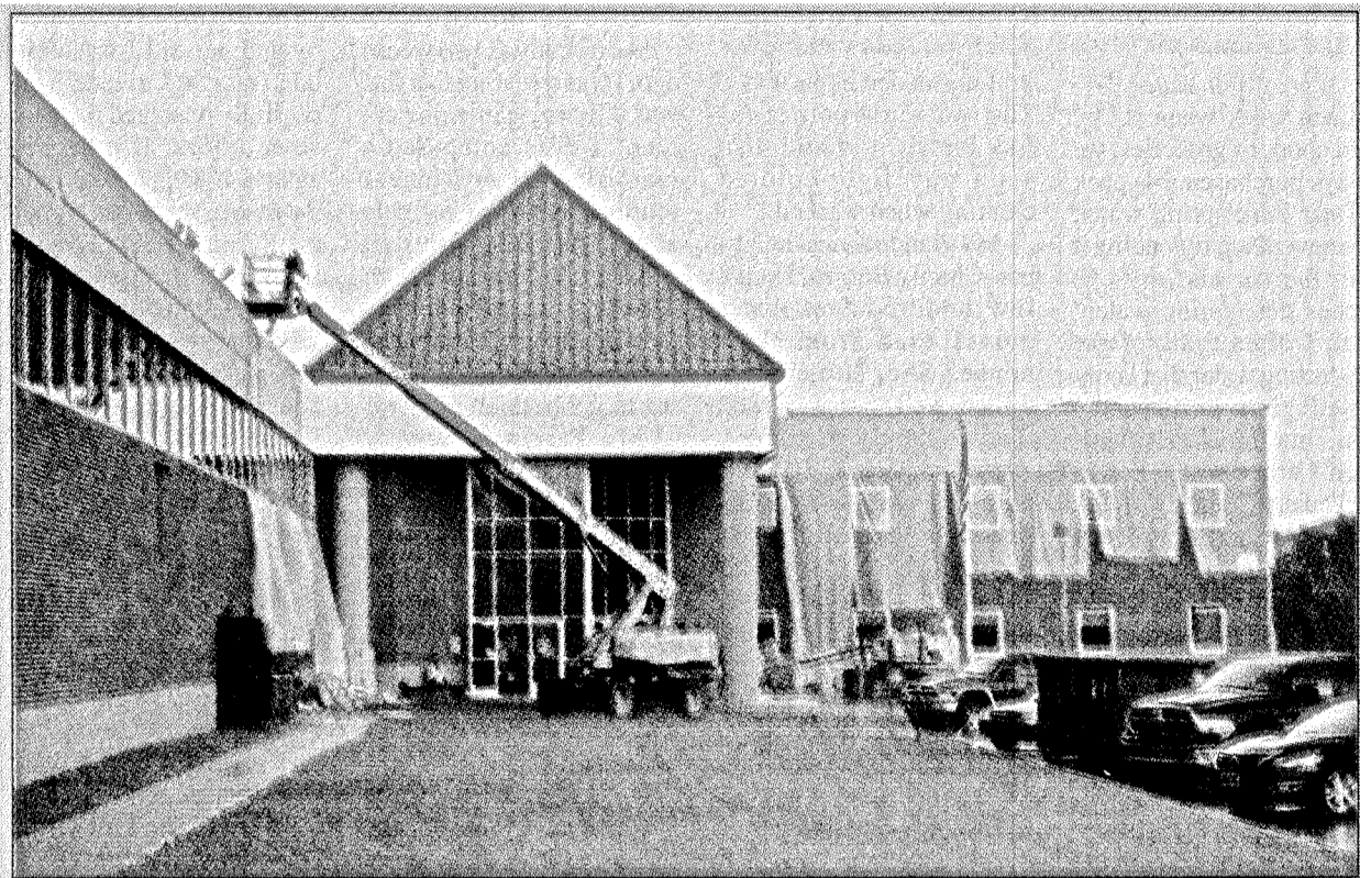
Trent Clark, Director of Facilities for Rockcastle County Schools, told members of the Rockcastle County Board of Education, at their last meeting, that work at RCHS is on schedule and, barring any unforeseen events, classes should begin as scheduled on August 15th. Clark said there were a few slight rain delays in early summer, but the work is still on schedule. Clark said he is working closely with contractors and work on the new front entrance and the heating and cooling systems, as well as other smaller jobs at the school, is progressing.
