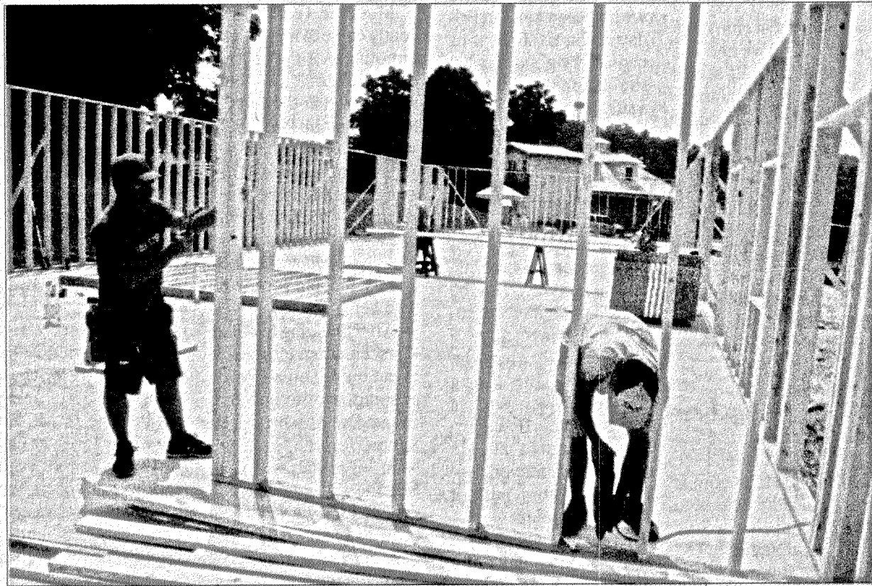
Workers for the McKeehan Construction Company started placing interior walls last week at the new Farmers Market on Richmond Street. The concrete pad is complete and officials hope to open the building for business before the end of the growing season this year.
