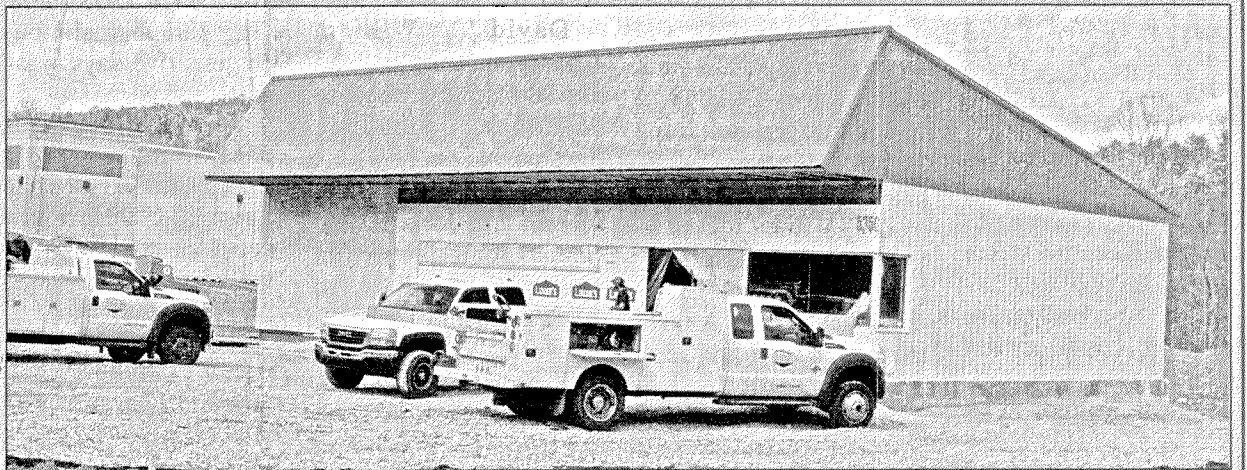
The new Marathon station in Livingston is now under roof and owners are still planning to open for business by Memorial Day of this year. Mayor Jason Medley said the new business will make a noticeable difference to the citizens of Livingston and will provide a convenience that the city has been missing for many years. The station is next door to the new Family Dollar store which opened last year.
