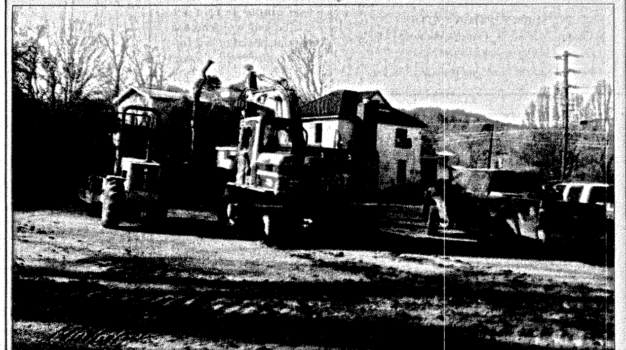
Goff Excavating of Mount Vernon has started the sitework for the upcoming Farmers' Market facility on Richmond Street. The house on the property, in the background, is also being demolished to make room for an entrance and more parking.
