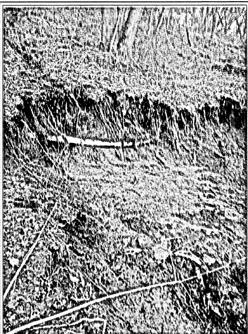
A six-inch water main near Livingston was exposed and broken due to recent mudslides causing 40 customers to be without water for several days. However, crews repaired the line and now Livingston customers are under a boil water advisory until further notice.
