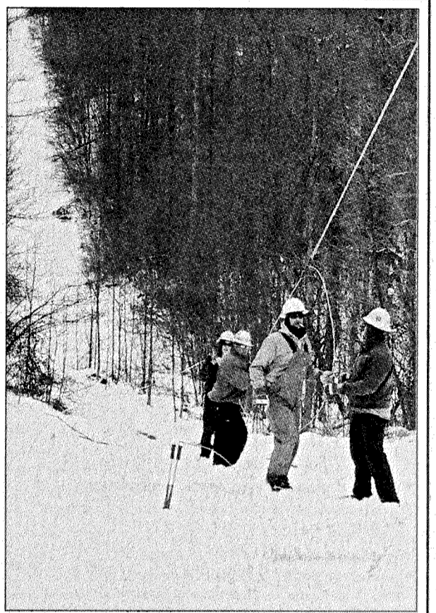
Jackson Energy Line Tech Brent Arvin works with crews from the Davis Elliott Company to restore power following last week's snowstorm.
