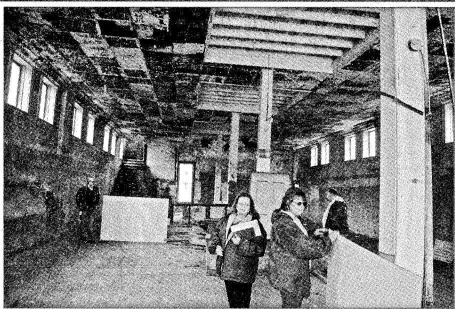
RTEC Executive Director Shirley Cummins, forefront left, and Procurement Management Director Freda Parsons, spent part of the day Tuesday going through the Jones Building and making plans for the upcoming renovations. Other members of the renovation team explored the building as well getting ideas for possible uses of the structure.
