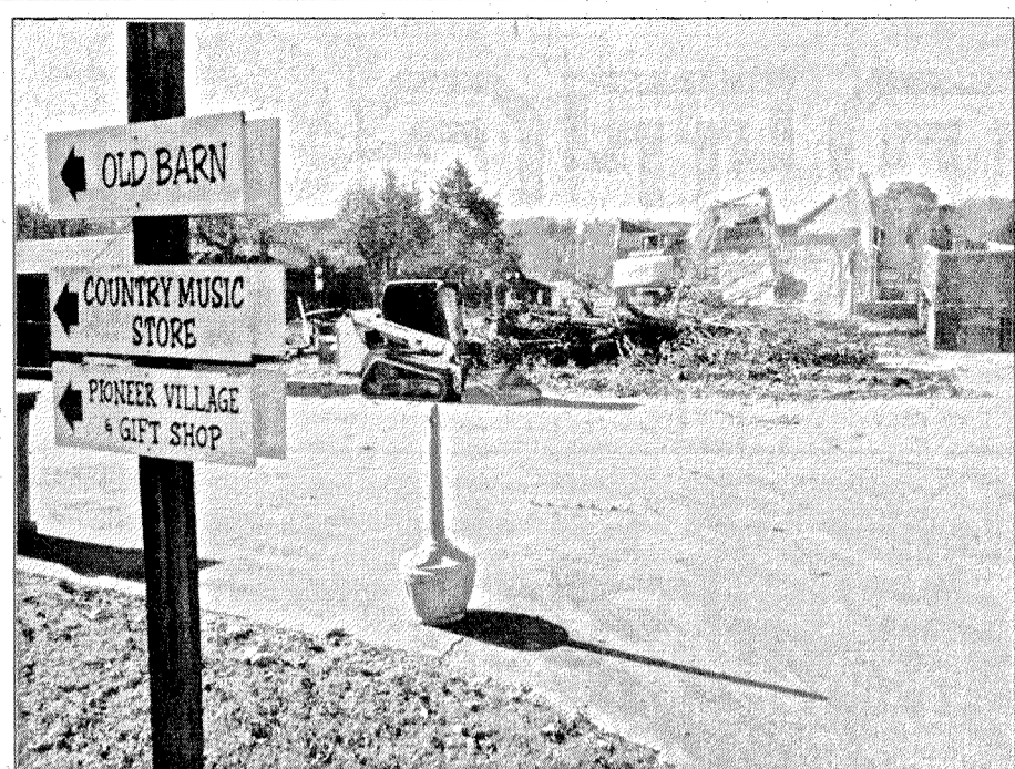
Crews were seen Tuesday demolishing one side of Renfro Village. Officials say owners are planning renovations for the area and have plans that are expected to bring even more tourists to the area. Renfro Valley has been a major attraction in Mount Vernon for over 75 years as the entertainment complex broadcasts the Sunday Morning Gathering in many countries around the world.
