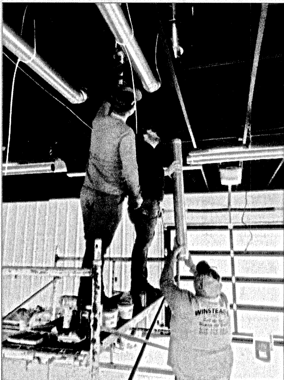
Winstead's Heating and Air work to install propane heaters in the market area of the new Farmers' Market on Richmond Street. Officials say the new facility will open immediately after the paving work is complete.
