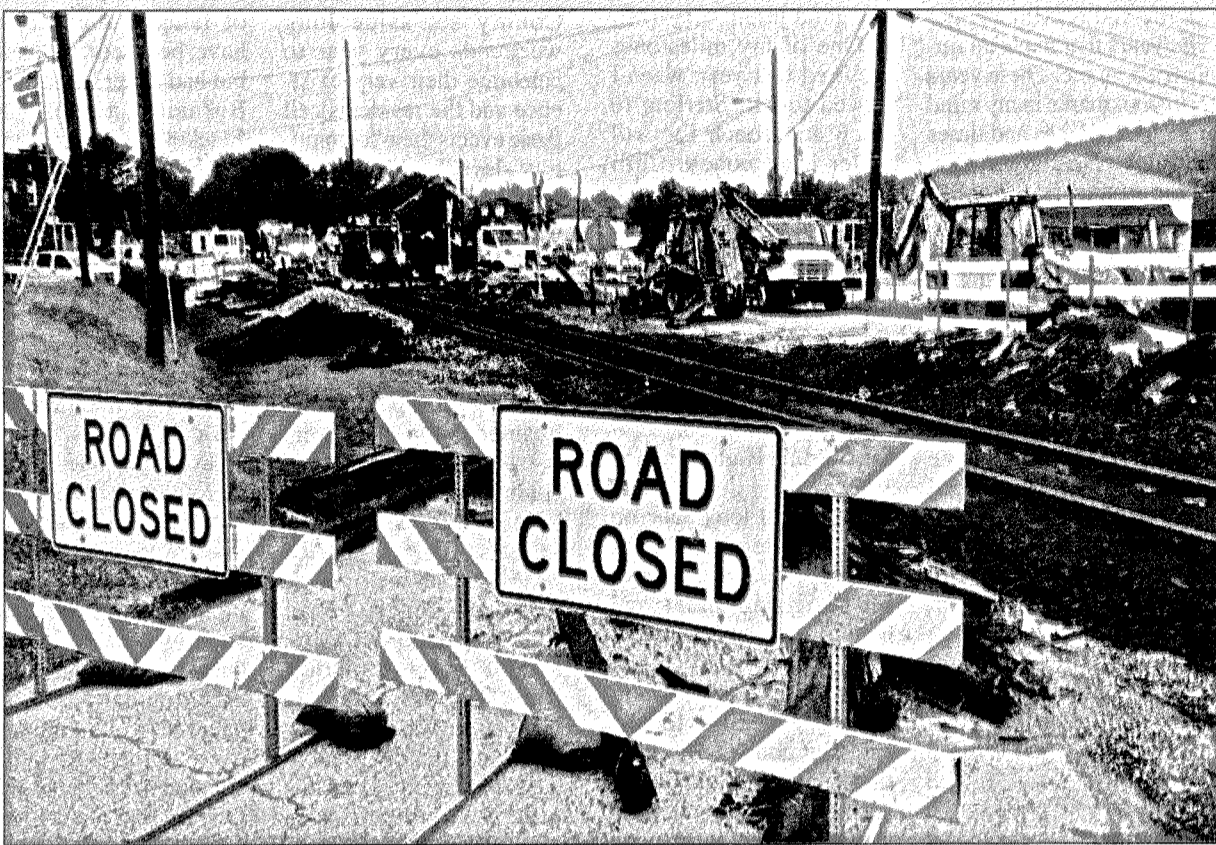
The southbound exit ramp at exit 62 was closed this week as part of the I-75 widening project and large equipment is prevalent in the area. Police are keeping an eye on the traffick and warning motorists of the roadwork near the interstate. The ramp is expected to be closed for more than four weeks. Several other roads in the city and the county were closed this week due to railroad crossing work and ramps at exit 59 are also under construction. Trucks are also entering and leaving the highway at the new Microfoodery plant on Richmond Street while it is under construction and some equipment is present on West Main Street for the ROOTS Project.
