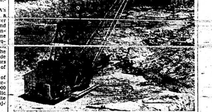
UNTIL LAST NOVEMBER the area where this dam is working was a part of the Tennessee river bed at the TVA's Kentucky Dam site. One of the greatest works of man created in dam construction this area, which covers about 40 acres. This giant dam removes six cubic yards of material at a bit.
