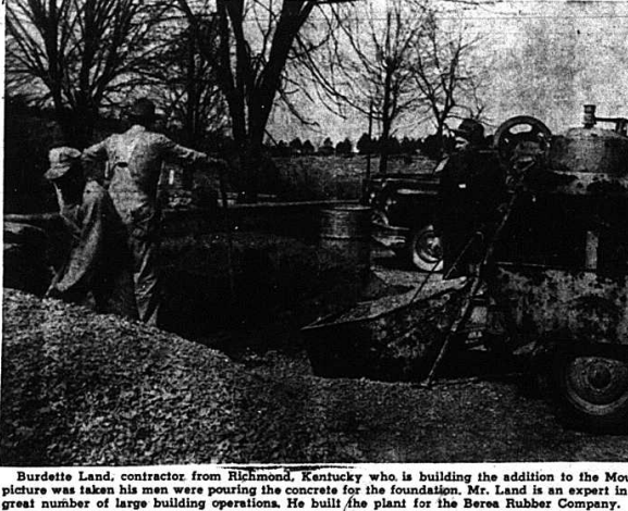
Burdette Land, contractor from Richmond, Kentucky who is building the addition to the Mount Vernon High school. As this picture was taken his men were pouring the concrete for the foundation. Mr. Land is an expert in construction and has handled a great number of large building operations. He built the plant for the Berea Rubber Company.
