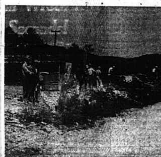
Members of the Coddell Construction crew drilling holes for blasting away the rock near Burr.
