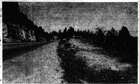
The U. S. Highway 25 just outside the city limits where drillers have been busy drilling holes for blasting away the ledge of rock on the south side of the road. This is to make way for the truck lane to be built up the hill. The wooden pegs used to plug up the drilled holes are hardly visible in the picture.
