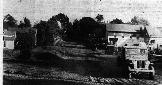
Main Street as it appeared last week. All the pavement has been removed and grading is being done. The street has been widened. To the right is the garage of Mack Bales.
