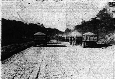
Truck loads of rock ready to unload into the spreader on the new highway U. S. 25 at Calloway. These trucks are hauling the foundation rock from the Kentucky Stone Company in Mount Vernon. Favorable weather has greatly enhanced the progress of construction.
