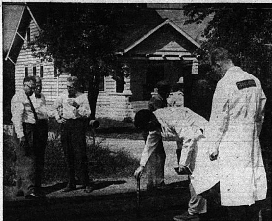
UNIVERSITY AIDS IN RUBBERIZED ROAD EXPERIMENT—Installation of asphalt pavement containing a newly developed synthetic latex compound, has been completed at Shively, Ky., on a three-mile section of the Dixie Highway. The work was done by the Kentucky Department of Highways. Combined with ordinary asphalt was a rubber latex compound developed by the Firestone Tire and Rubber Company through a research program being carried on for the company by the University of Kentucky Research Foundation. The installation on the heavily traveled route is expected to show to what extent the rubberized material is more durable and flexible than ordinary asphalt surfaces. Above at the left are Carl Shaffer, Firestone executive from Akron, Ohio; D. V. Terrell, dean of the University's College of Engineering and director of research laboratories for the Kentucky Department of Highways; and L. E. Gregg, assistant director of research for the Department of Highways. A Kentucky Research Laboratory technician and a Firestone engineer are shown testing the thickness of the surfacing.
