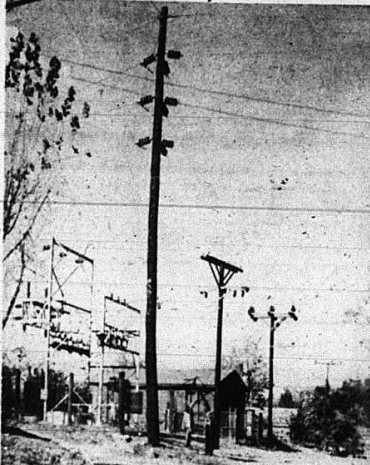
A new pole installation at the Mt. Vernon substation of Kentucky Utilities Company is pointed out by Roy B. Owens, K. U. manager.
