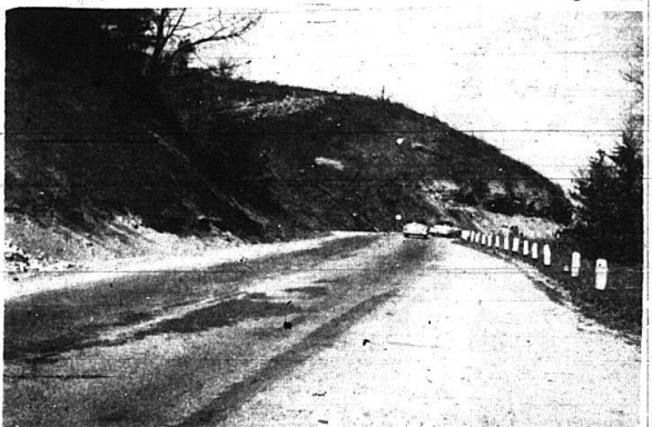
Looking north at the Boone Gap Hill through which the new U. S. 25 will lead. The cut will be 103 feet at its greatest depth. The picture was taken last Tuesday after the clearing crew had cut down all the timber on top of the hill. Road machinery is now at work gouging on the hill. — Photo By The Signal
