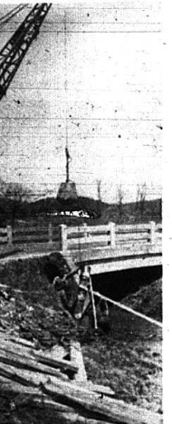
The derrick that is used to pound the posts for the drive in bridges that are built to route traffic over past the place where a new bridge is being built. The derrick is lifting a 3,000 pound steel ball which is also used to break down the old concrete bridges. PHOTO BY THE SIGNAL
