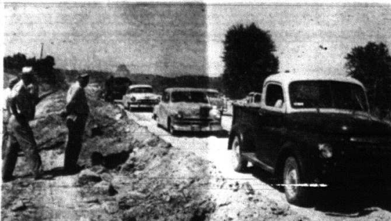
Part of the highway near Snider where grading is almost completed and where the pouring of the concrete foundation started this week. The picture shows a line of traffic as it moved slowly over the new grade.
