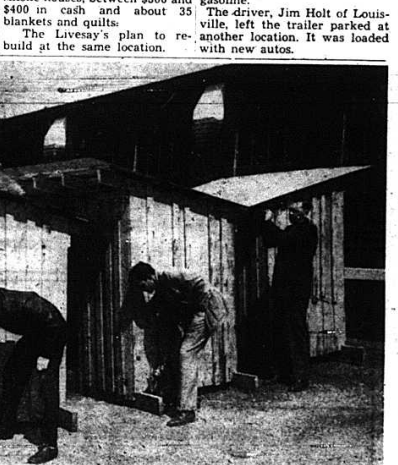
SHELTERS for school children waiting for school buses in Rockcastle County are nearing completion by the Mt. Vernon Jaycees on Richmond Street. When completed there will be 11 shelters through the county. Shown at work on the shed houses are, left to right, Joe Henderson, Earl Watkins, Charles Baker, Warren Ferguson. On the roof is Shannon Franklin.
