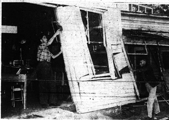
PUSH BOYS —Dave Burke, right, and W. D. Scaggs, clean up the area after an auto driven by Cecil Towary. Towary was injured, but the store suffered an estimated $100 worth. The property is on S. E. 25 east of Mt. Vernon and was once a tourist, court owned by Jim Winstead. Residents described the crash as "like an earthquake."
