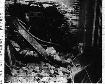
DRIVE-IN BANK —This hole, about eight feet in diameter, was knocked in the wall of the Citizens Bank at Brodhead about 1 a. m. Wednesday by a truck loaded with coal. The truck's driver, 23-year-old Marvin Sizemore of London, said he lost control when he met two cars as he turned the corner near the bank. Officials declined to estimate damage to the bank.
