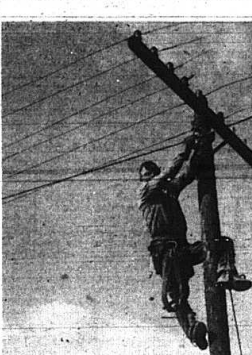
A REAL LIVE WIRE—Joe Adams, manager of Northeastern Telephone Company in Rockcastle County, relates a wire to a pole, having the wire cut by workmen to trim an interfering tree. The wire is carrying current.
