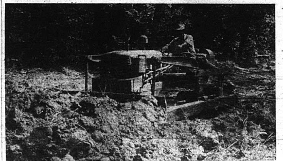
UNDER CONSTRUCTION—Residents of the Buckeye, Hummel and Wildie communities are working together to get a two-mile stretch of road to Maret Cemetery. Pictured above is Henry Bluff operating a bull dozer belonging to Elmo C. Anderkin. On another section of the road a crew of men are drilling and blasting.
