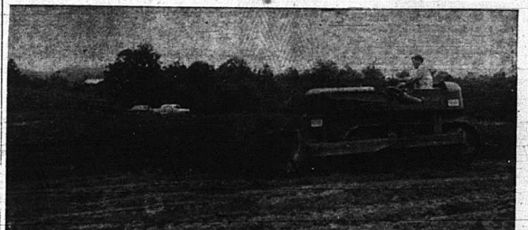
CONSTRUCTION WORK has been underway at the Livingston playground for four days. Only one more days work is required to complete the building. The dozer pictured is owned by Elmo C. Anderkin. The operator is Guy C. Martin.
