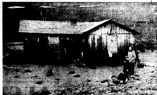
HOME of Mr. and Mrs. Buster Northern, in northwest Brodhead was carried about a quarter-mile down the Dix River and deposited in a field. The house was split open and the contents destroyed. No one in the Northern family was injured.
