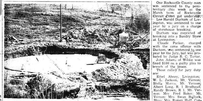
SEWER PLANT - Despite off and on bed weather, work is underway on the city's new sewer disposal plant on Town Branch at the end of Newcomb Avenue. Considerable concrete has been poured by Tye and Walls, contractors from Eminence. Installation of sewer lines is expected to begin about the middle of March.
