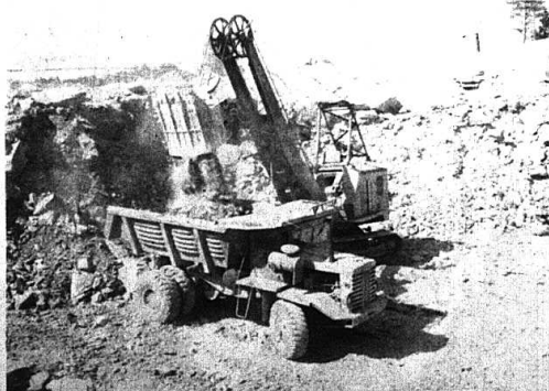
LIMESTONE AND DUST - Two ingredients in all road building in Rockcastle County are limestone and dust. Shown above is a shovel loading a dump truck and stirring-up both. The shovel is in the area of Hayes Cut just south of Conway. This section of the new superhighway is not expected to be opened until late in the summer of 1967, if then.
