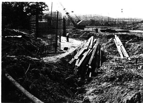
ONE OF THE UNDERPASSES - Workmen are shown constructing framework for a concrete underpass on Lambert Road between Boone and Snider. The underpass is near the farm of James H. Lambert, Sr.
