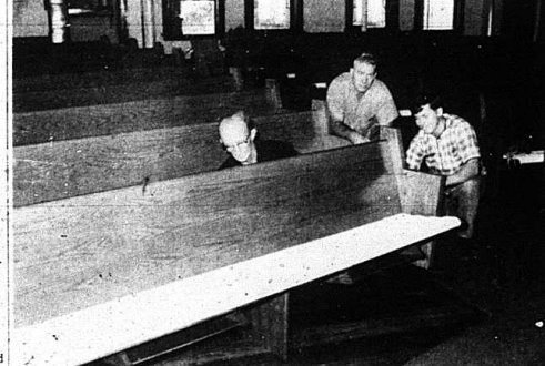
A SOFT SEAT —Those who attend a revival beginning Sunday night and continuing for two weeks at the Mt. Vernon Christian Church will have a soft seat on which to sit. Above, workmen install new pews at the church this week. The 30 pews will seat about 200 persons. They are almost up veneer with cushions. The church also purchased a match-pull communion table and chairs. Installing the pews are Floyd Yant and Don Scott of Warsaw, Ind., with Walker Hines of Mt. Vernon in the background.
