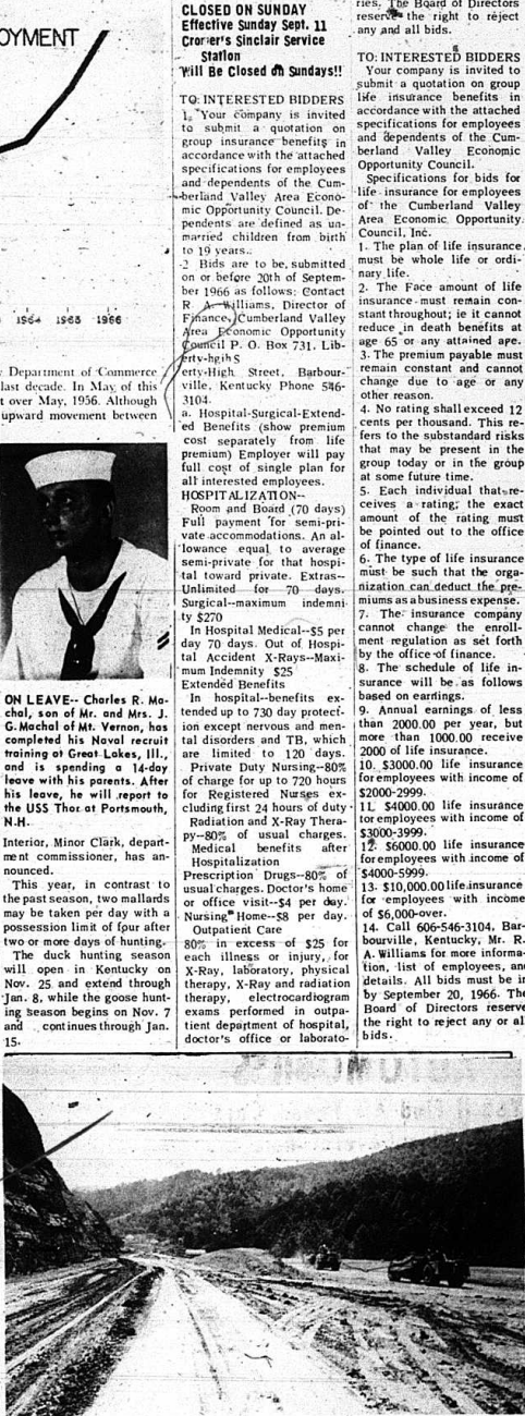
SMOOTHING THE WAY for a new U.S. 119 near Harlan keeps these earthmoving machines busy. State-Highway Commissioner Henry Ward said the route is to be rebuilt from its beginning on U.S. 25 at Pineville to the West Virginia border in Pike County, where it crosses Turk Fork. The job is part of the Appalachian Development program, which will provide 435 miles of developmental highways in Eastern Kentucky.
