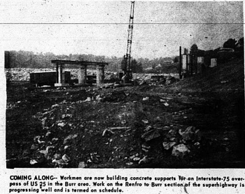
COMING ALONG —Workers are now building concrete supports for an Interstate-75 overpass of US 25 in the Burr area. Work on the Renfro to Burr section of the superhighway is progressing well and is termed on schedule.
