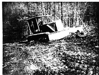
This D-6 B Catipilar tractor with improved hydraulic fast drop blade to speed up work while clearing land or grade work, has proven a good work horse for any type bulldozer work that comes along.
