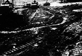
Anderson and Martin Construction Company are in the process of building a 35 foot dam on Indian Lakes Farm owned by David Graves of Lexington. The dam will back up water to form an approximately 16-acre lake. The trees shown in the background will be the water-line.
