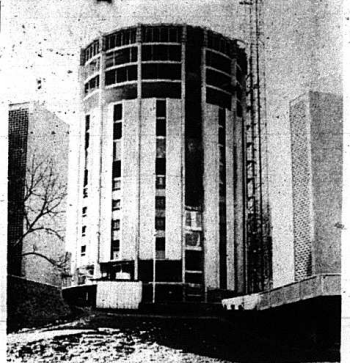
MIGNON TOWER GOING UP —This is the fourth in a complex of women's residence halls at Morehead State University. The others are completed and occupied. The new tower will accommodate 300 students, making a total of 1,004 for the entire complex. Completion of the 16-story tower, named for Mrs. Adron (Mignon) Doran, wife of Morehead's president, is expected in June. Cost will be $1,540,000.
