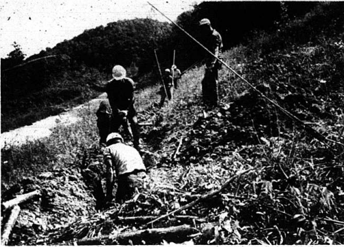
In the above photo, a crew of Jackson County R.E.C.C. is burying electric cables where the 175 bridges will between Rockcastle and Laurel Counties.
