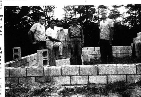
LENDING A HELPING HAND - seems to be the order of the day as Bro. Norman Howard, extreme left, Joseph Hansel, Russell Ramsey, and Bro. Larry Johnson, contemplate the block work began on a cabin being built at the Kentucky Christian Churches camp site. According to Bro. Howard, all block will be laid Saturday when several volunteers will converge on the camp to help with the job.
