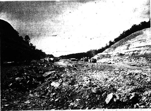
CUTTING IT DOWN TO SIZE. —The Chestnut Ridge section will soon have a different look entirely as work on I-75 progresses rapidly. Rock from the mountain is being used to fill the hollow to the north of the cut.
