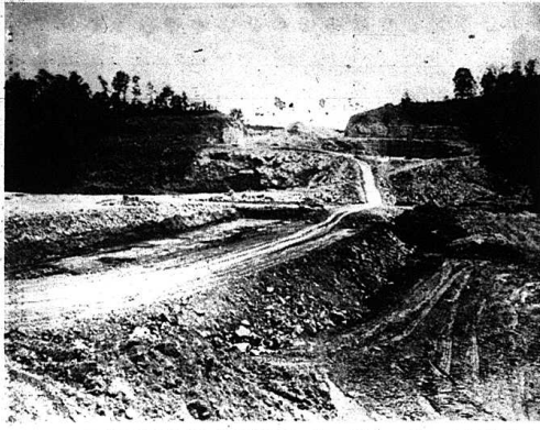
LAKE AND HIGHWAY GO TOGETHER —Construction of Interstate 75 takes the form of a dam two miles north of Mt. Vernon to create a 370-acre lake, scheduled to be completed next year. The highway-fill dam (center, foreground) will be built up and the lake will occupy the area at the right to provide water for Mt. Vernon and for industrial, agricultural and recreational uses in the area. Sections of I-75 from Berea south and Williamsburg north will open this year. All but 15 miles of the 191-mile route from Covington to the Tennessee line near Jellico are now under construction.
