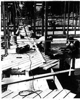
BOAT SLIPS FOR KENLAKE —One hundred covered boat slips, now under construction at Kenlake State Park near Hardin, are slated to be completed and ready for use by this fall to meet the growing demand for storage and servicing created by an increasing number of boats in the Kentucky Lake area. The $165,000 project is being financed by revenue bonds.
