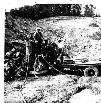
SEEPAGE CONTROL. —A crew from Felix and Sison Co. of Oklahoma are shown drilling 2½ inch holes some thirty feet deep and filling them with concrete under pressure at the site of the dam at Renfro. The holes are being drilled to prevent water seepage to the core of the dam. When this picture was taken (Wednesday) there remained about 12 foot of dirt to be removed down to rock.
