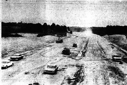
PROGRESS ON PURCHASE PARKWAY—Grade and drain on the entire 57-mile Jackson Purchase Parkway is 82 per cent complete says State Highway Commissioner Mitchell Tindler and all of the paving contracts have been awarded. This stretch of the superhighway is under construction just north of the U. S. 68 interchange in Marshall County. The route runs from the Tennessee line near Fulton to an eventual junction with I-24 between Paducah and Kentucky Dam Village State Park.
