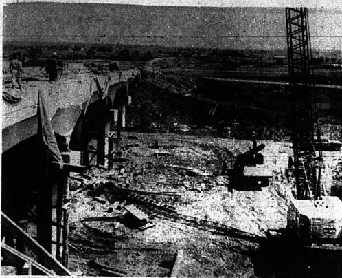
INTERCHANGE CONSTRUCTION ON I-65 —Construction moves ahead on the interchange where Ky. 70 crosses I-65 near Cave City in Barren County. State Highway Commissioner Mitchell W. Tinder says the interchange will be open for travel by the fall of 1968. More than 100 miles of the superhighway, between Louisville and the Tennessee border are already open to traffic.
