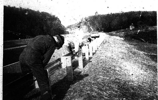
175 BY-PASS OPEN? According to Emmett Roberts of the State Department of Public Information there is a possibility that the Interstate 75 By-Pass from Renfro Valley to Bere will be opened in time for Christmas traffic. The guard railing is installed except that which goes on the end and that is possibly the most important section. A decision will be made Thursday morning (today) on whether to open the section or not. Mr. Roberts told the Signal. Workmen are shown putting the final touches to the railing in the above photo. If the by-pass is opened in time for the Christmas traffic from the north, plans are to ask road stations in Cincinnati and a little further south to broadcast the information so that motorists may use it. No opening ceremonies are planned by the State Highway Department.
