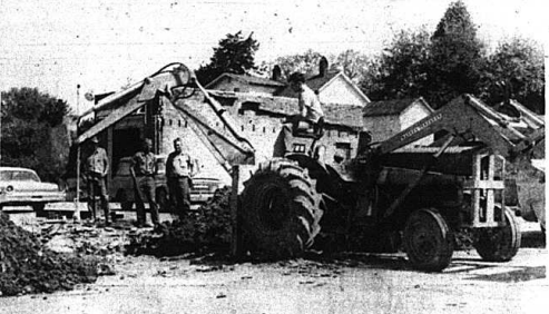
PEPPER STATION--Work was begun Wednesday on a pepper station for Rockcastle County. The station will be located on US 25 just south of Mt. Vernon at the old Hall Way House site. In the above photo, William Lewis Barrett, operator of the back hoe is digging a pit for truck scales. Looking on from left is: Roscoe Bullock, Edd Hubbard, and Robert Hubbard, station manager.
