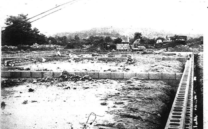
VOCATIONAL SCHOOL PROGRESSES—The Harry M. Sparks Vocational School, located on the old Brodhead Road, is well under way. A large amount of dirt had to be hauled in to bring the grade up to the proper level. Mays Construction Company of Williamsburg, one contractor for the $450,000 project. The Rock-
